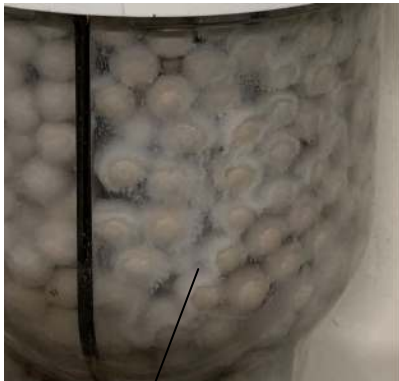
Figure 9: Salt precipitate deposited on neutralization media from Aluminum heat exchangers
